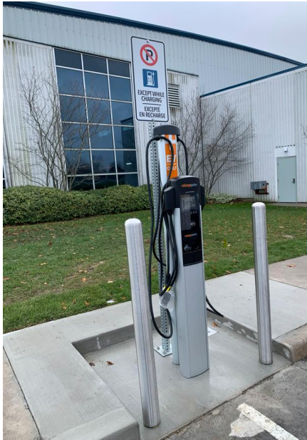
Figure 10 Level 2 EV Charging Station at McKinney Centre
