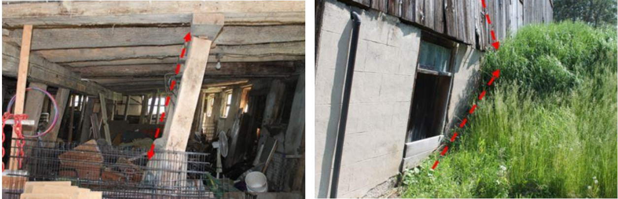
Figures 30 & 31: (left) View of the interior structural supports of the barn, looking east, (right) View of the south elevation noting the bowed foundation resting upon a pile of fill (Source: MHBC, 2023).
