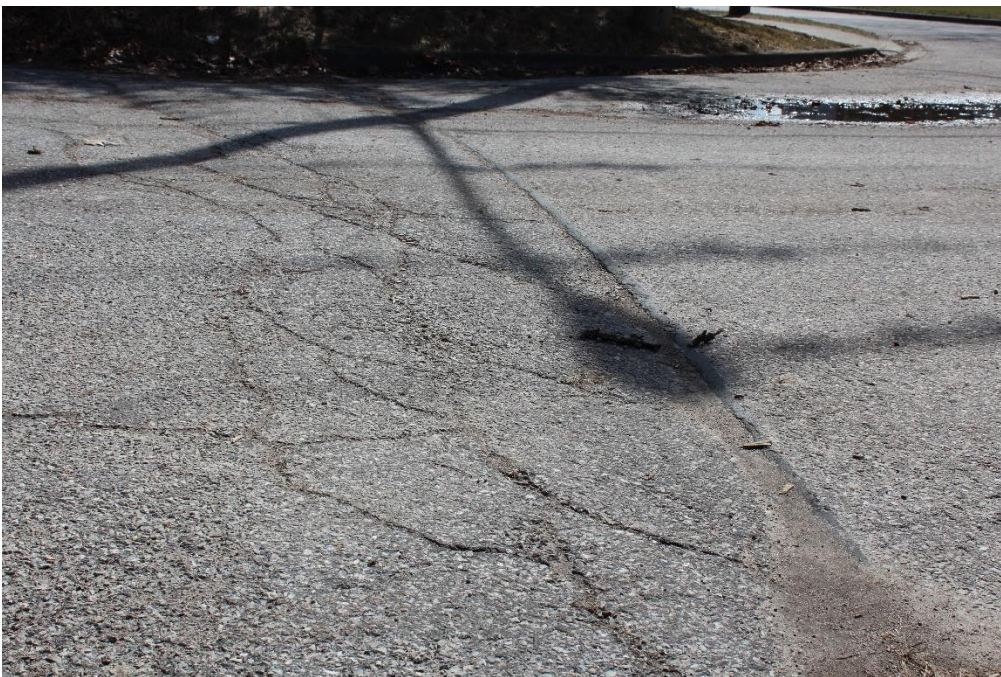
Figure 15 A photo of a road in Poor condition
