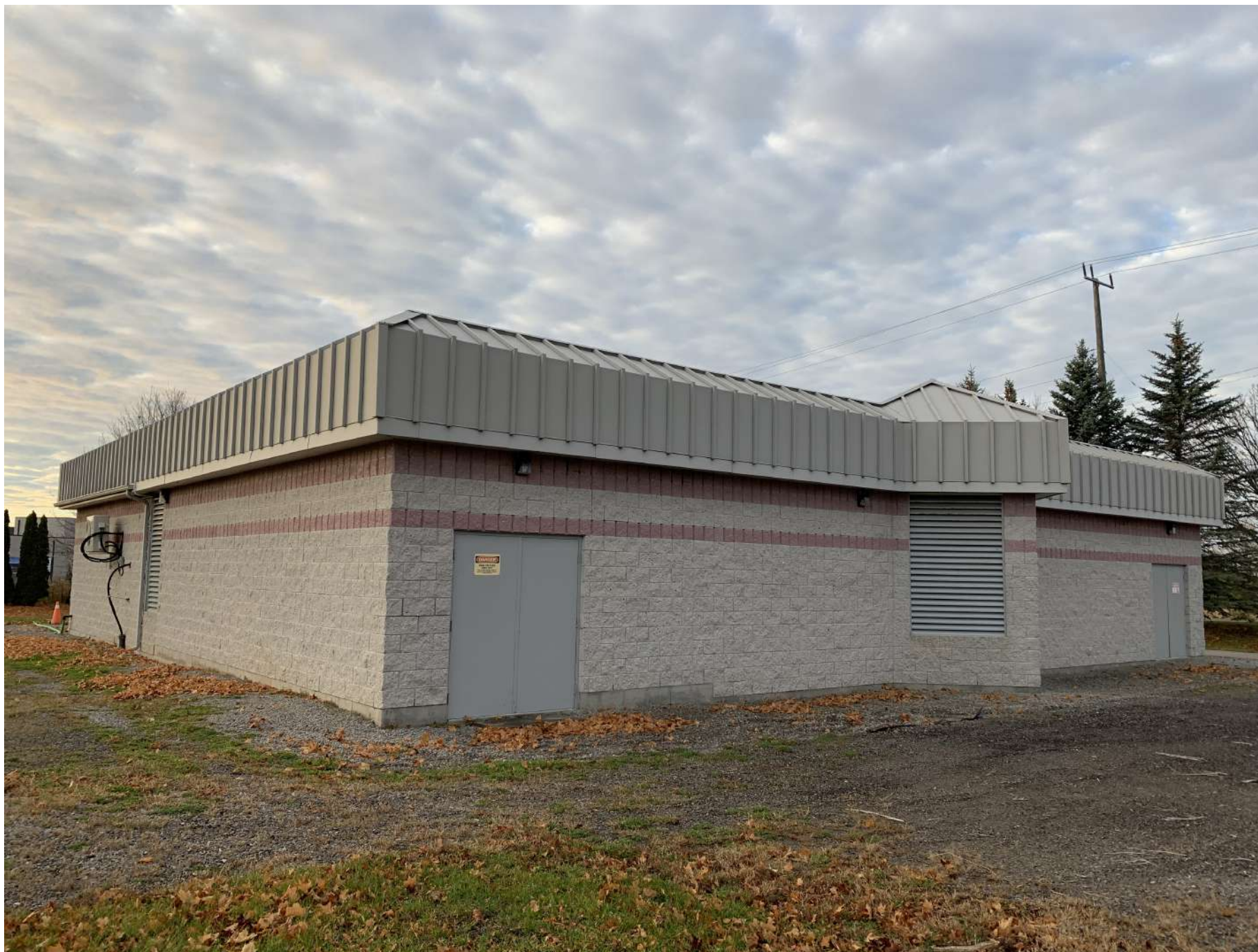
Picture of an enclosed electrical sub-station (Source: Elexicon Energy Inc.)
