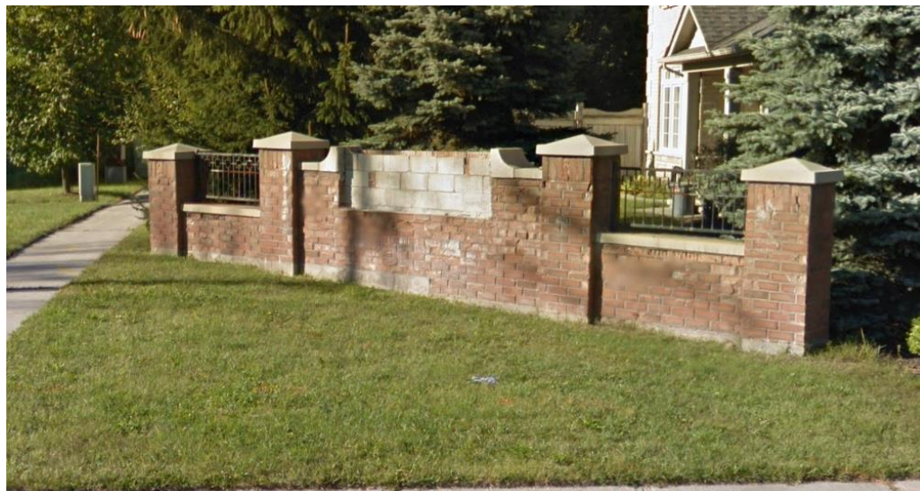
Anderson St and Solmar Ave – Damaged Masonry Feature 2014
