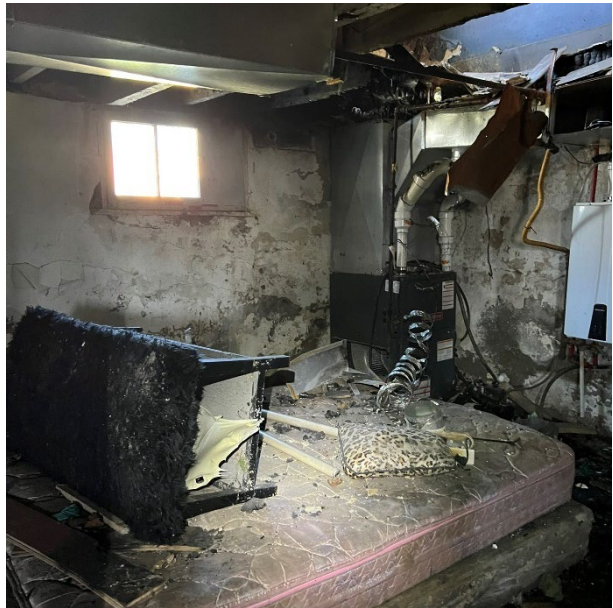
Basement with Fire / Fire Suppression Damage (Ceiling Collapse)
