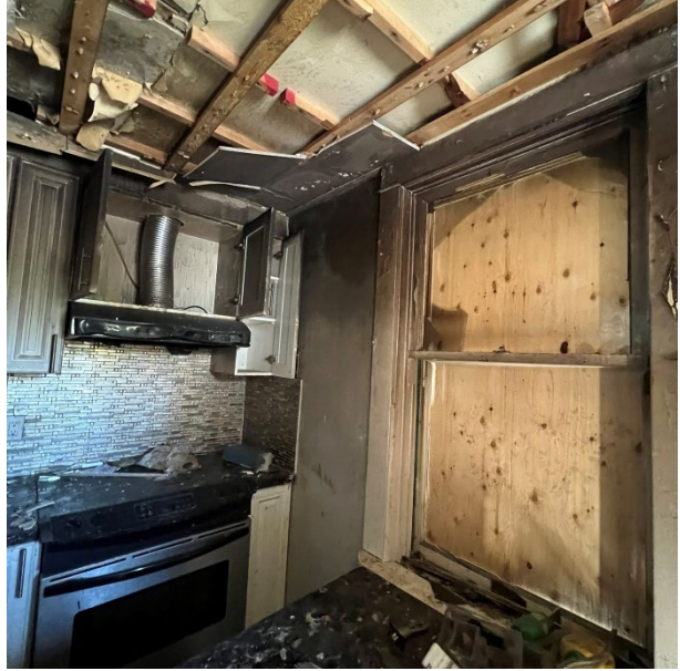
Kitchen and Fire Damage (Original Section)
