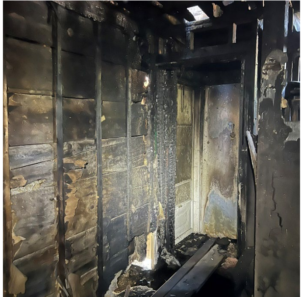
Rear Addition with Total Fire Destruction
