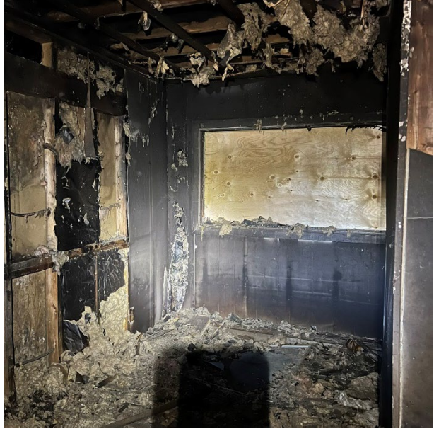
Rear Addition with Total Fire Destruction
