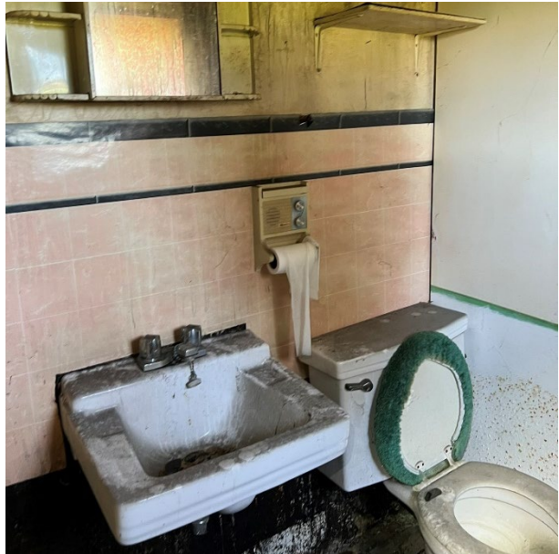
Damaged Basement Bathroom
