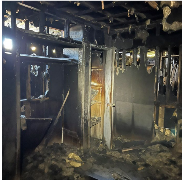
Rear Addition with Total Fire Destruction
