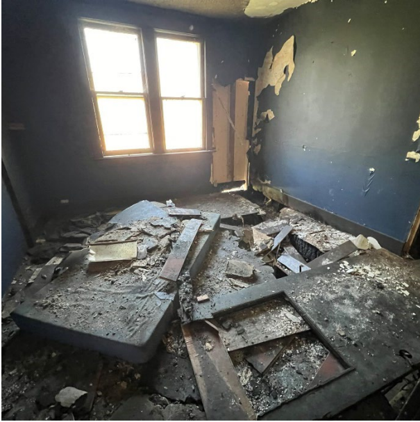
Room and Fire Damage (Original Section)
