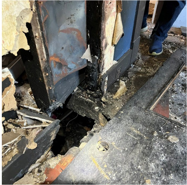
Burnt Through Walls and Structural Elements
