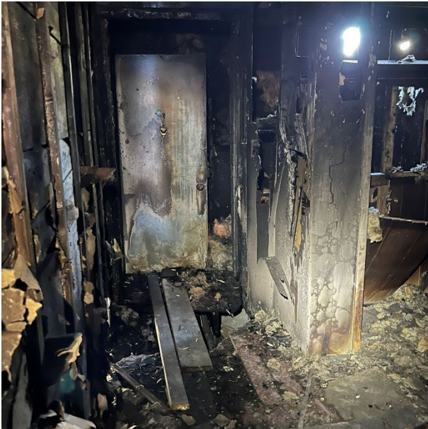
Rear Addition with Total Fire Destruction
