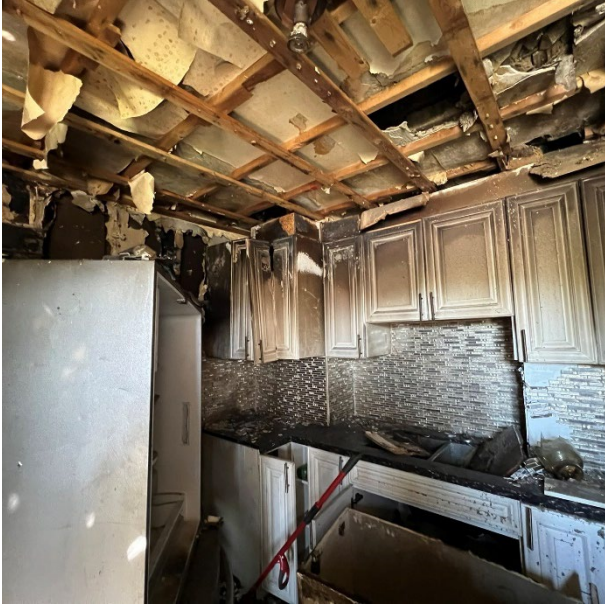
Kitchen and Fire Damage (Original Section)
