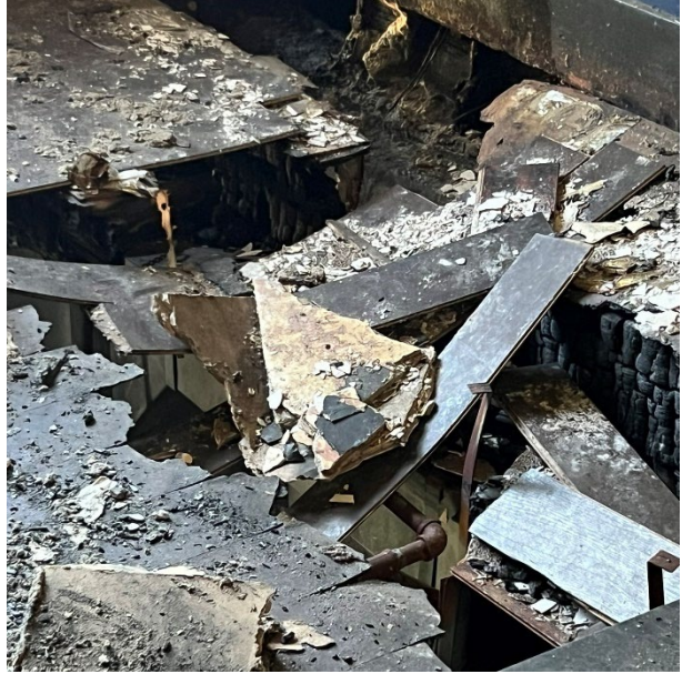
Burnt Through Floor (Original Section)
