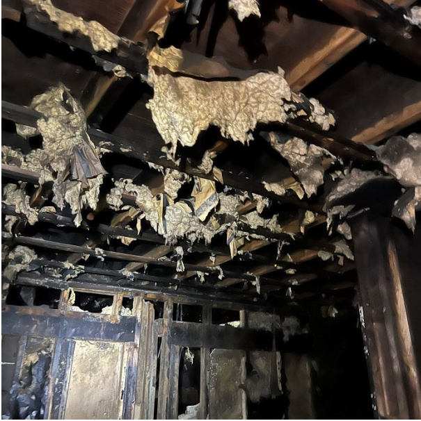
Rear Addition with Total Fire Destruction
