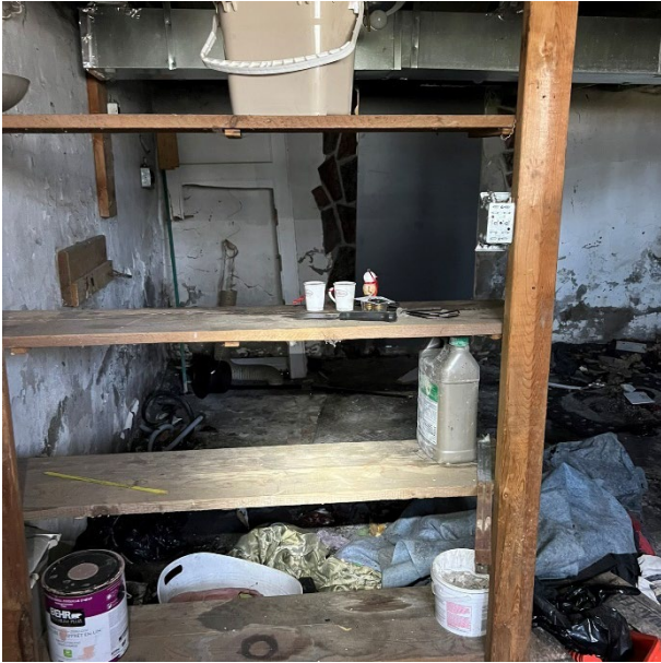
Basement with Fire / Fire Suppression Damage
