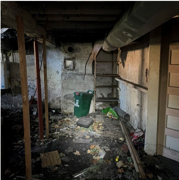
Basement with Fire / Fire Suppression Damage
