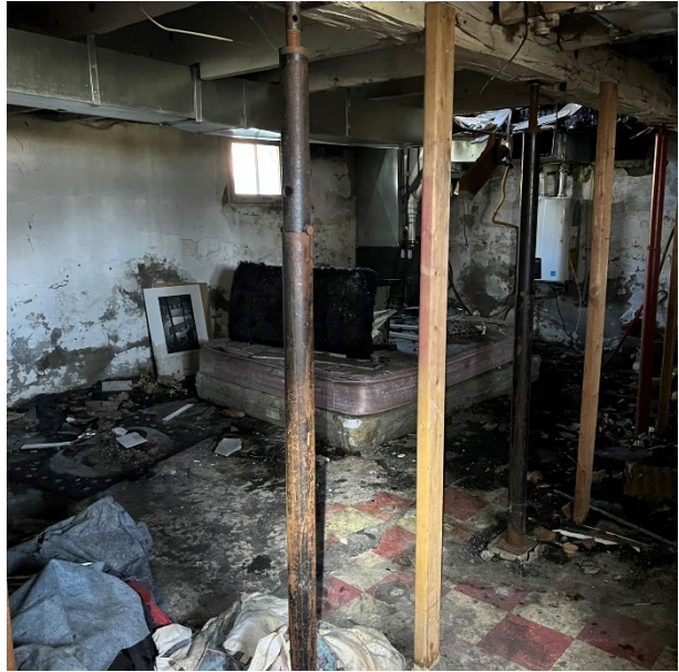
Basement with Fire / Fire Suppression Damage
